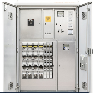
• METERING &amp; DISTRIBUTION
